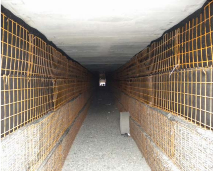
Large open chamber allows for accessible inspection and maintenance. Note: No movement/stress in the upper portion of the wall below the bearing sill.
