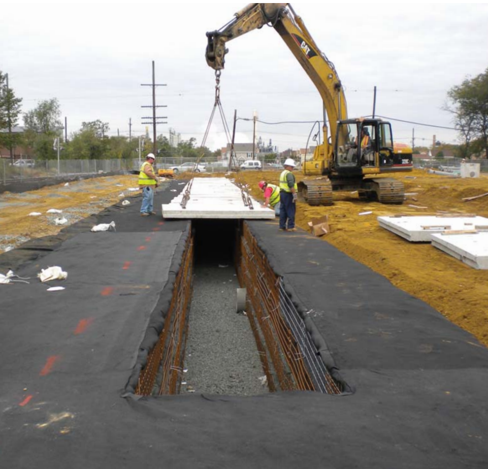
Precast roof deck panels placed directly on geosynthetic-reinforced walls. Design note: No concrete grade beam required on bearing sill.
