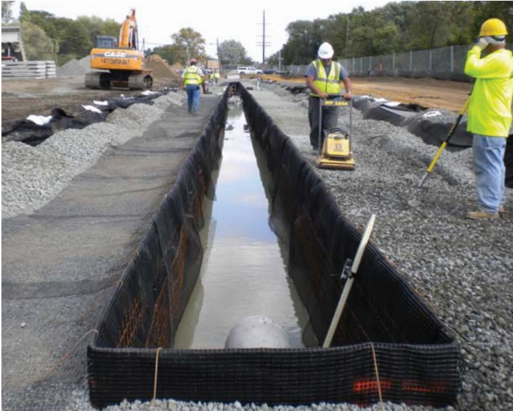
Geosynthetic-reinforced stone perimeter walls constructed with geogrids and compacted open graded stone.
