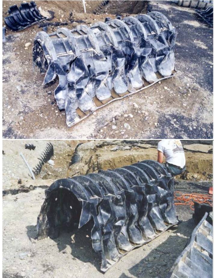
Figure 8. Recovery of deformation with time. The middle photo of Figure 7 shows the buckled shape when the arched filler was cut out; The top photo in this figure shows partial recovery of the deformation of one of the legs of the main chambers within a 1/2 hour after being cut out. The bottom photo shows full recovery of most of the deformation days after it was originally excavated by the contractor.
